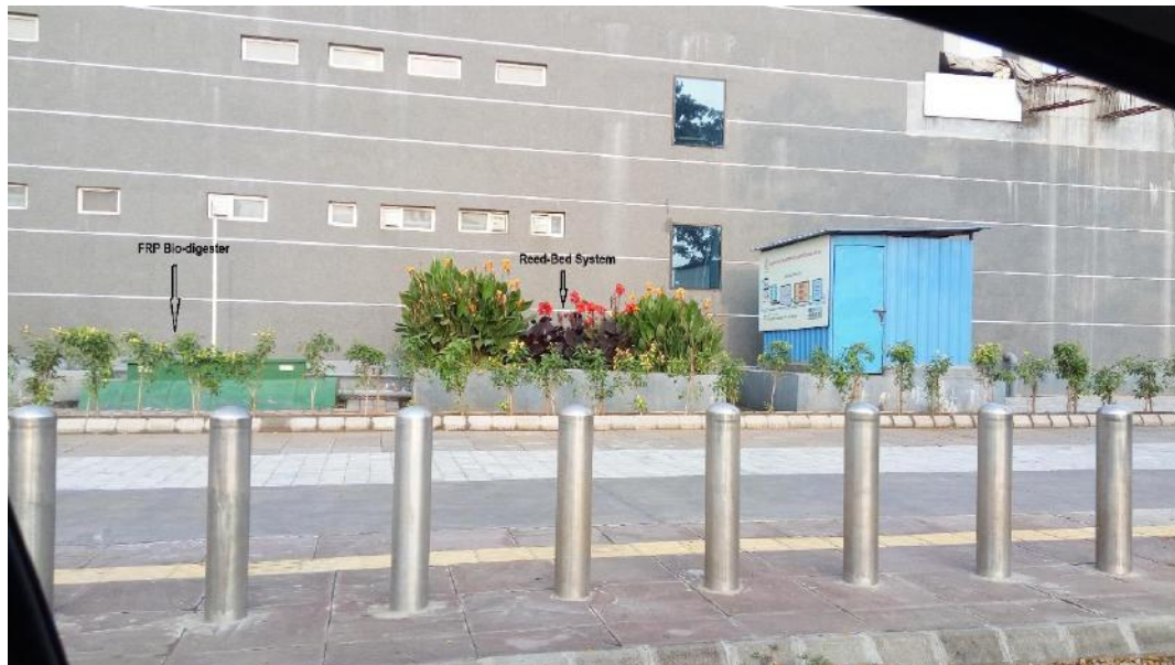
BIO-DIGESTER At Airport South station
