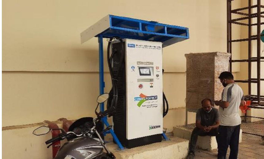
EESL charging station at Congress Nagar Metro Station
