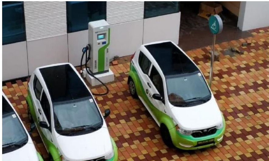
EESL charging station at Airport Metro Station
